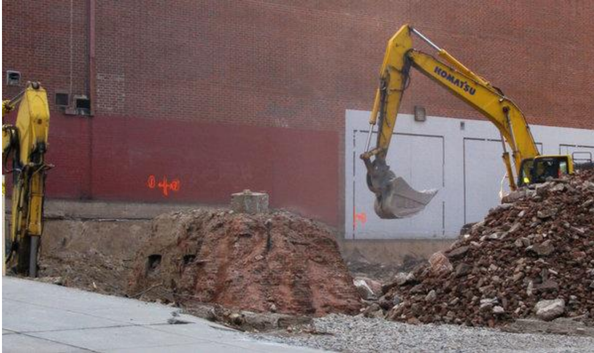
Excavation on East 92nd Street, between Third and Second Avenues, unearthed two arched openings below street level that were used for power or refrigeration by the Ruppert Brewery. Credit David W. Dunlap/The New York Times
